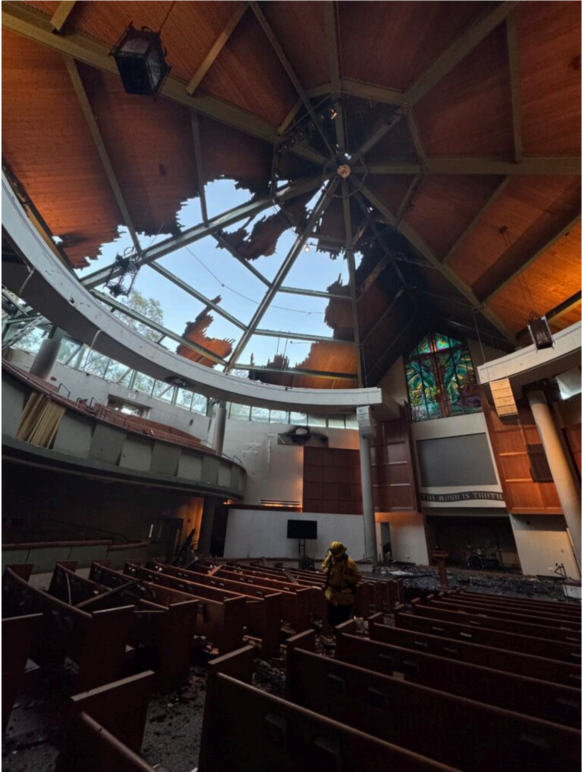
The Calvary Church Sanctuary was destroyed by the fire and subsequent rains.
